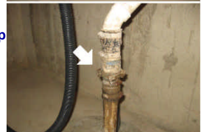
Sump Pump & Active Leak
