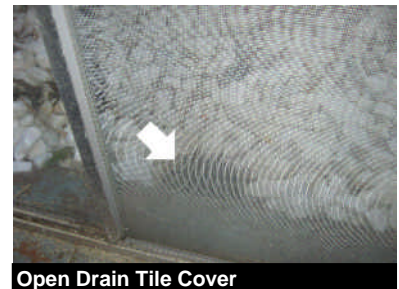
Open Drain Tile Cover
