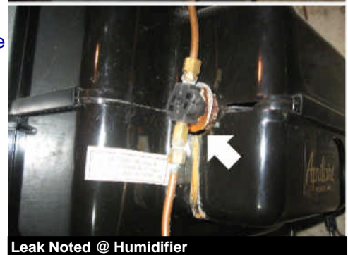
Leak Noted @ Humidifier
