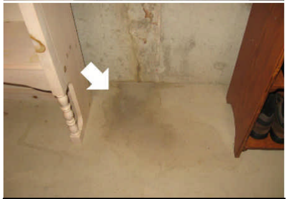
Evidence of Past Moisture Seepage
