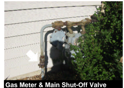
Gas Meter & Main Shut-Off Valve
