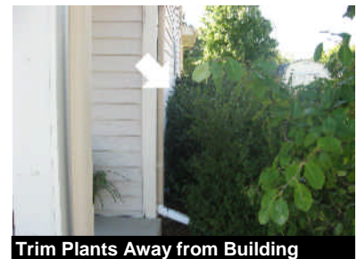
Trim Plants Away from Building
