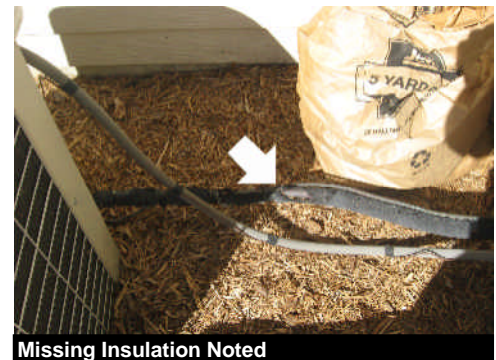
Missing Insulation Noted
