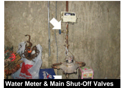
Water Meter & Main Shut-Off Valves
